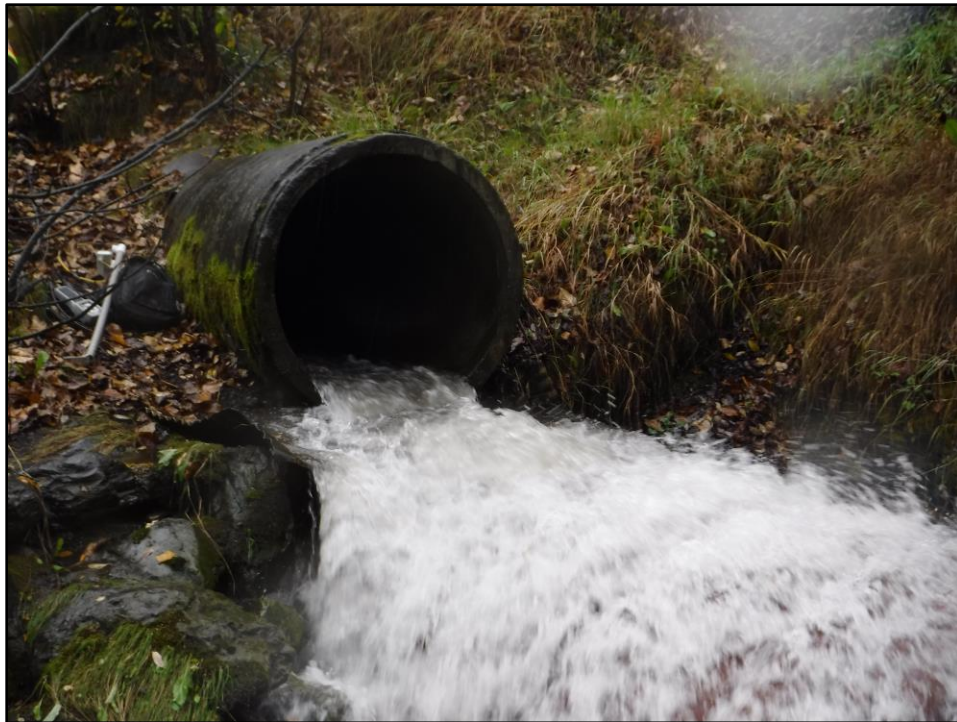
Photograph 8. Outfall SWM08 (86-1), New Seward Highway at Chester Creek.
