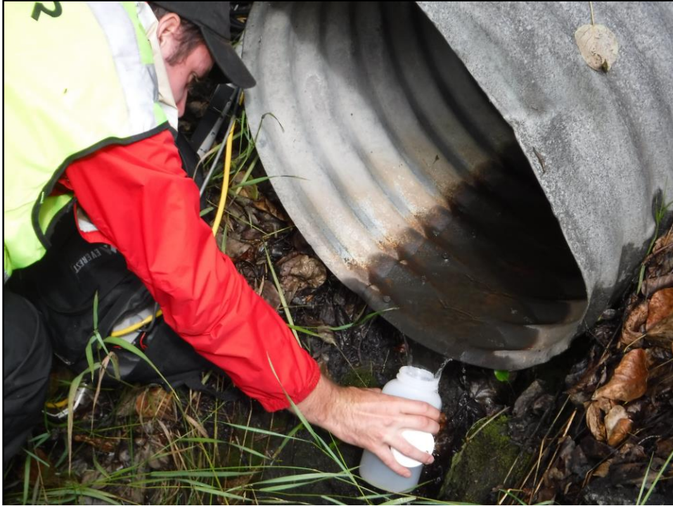
Photograph 7. Outfall SWM07 (484-1), New Seward Highway at Chester Creek.
